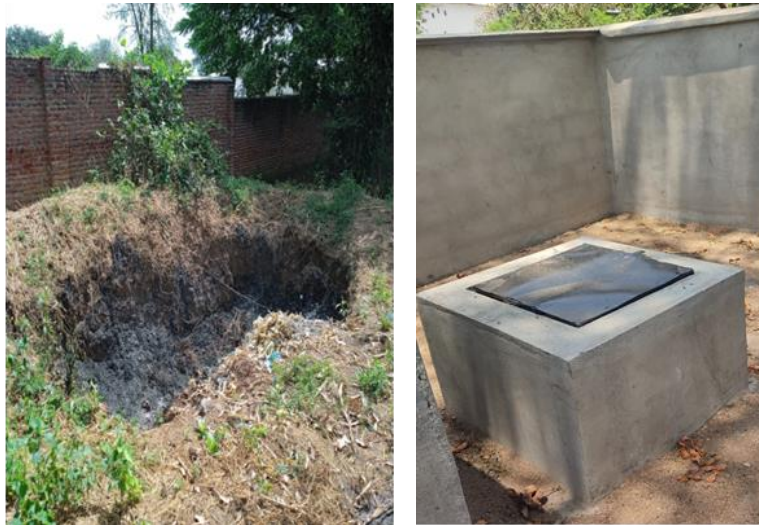
A pit that was used for disposing ash, left, and newly installed ash pit, right. Photo credit CRS staff
