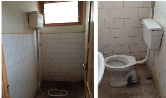
A toilet that was not accessible to people with disabilities, left, and new more accessible toilet, right. Photo credit CRS staff
