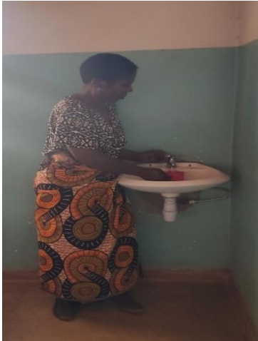
Your gift provided the Kankao Health Center with sinks to promote hand-washing and better hygiene. Photo by CRS staff
