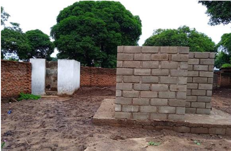
A newly constructed medical waste pit stands in the foreground. Behind it, the old pit is no longer usable. Photo by CRS staff
