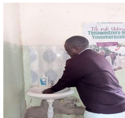
The Sister Martha Health Center now has better water and hygiene infrastructure. Photo by CRS staff
