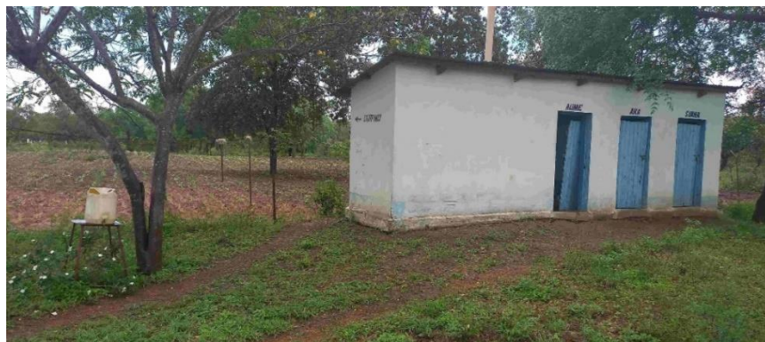
Old unhygienic toilet block that was out of use before this support. It had developed cracks in the slab and is being decommissioned.
