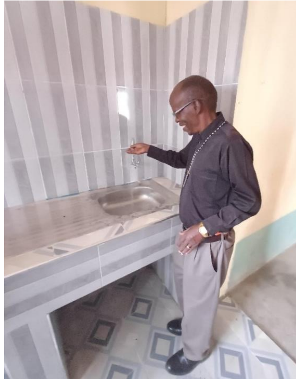
Father Benson Maluki (Facility Manager) checking the water flow in the newly constructed maternity bathroom.
